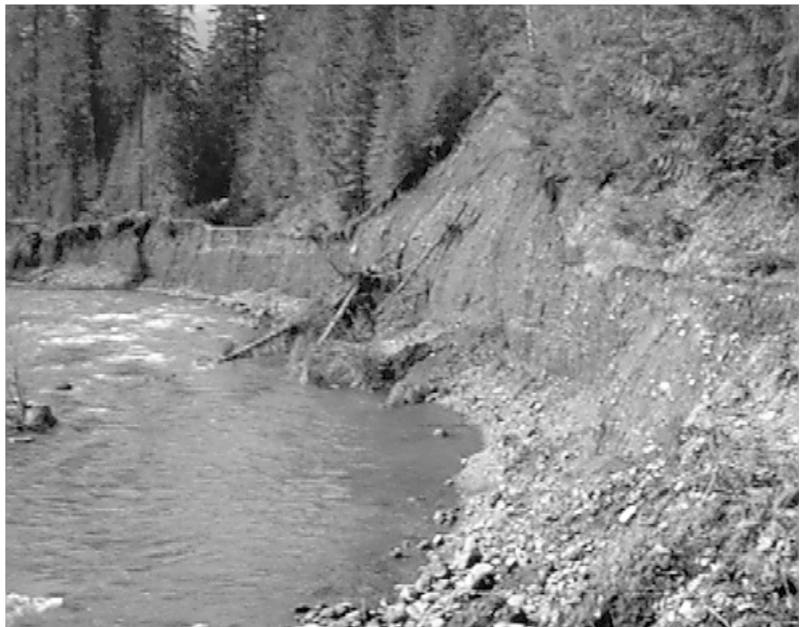
Dosewallips road washout.
